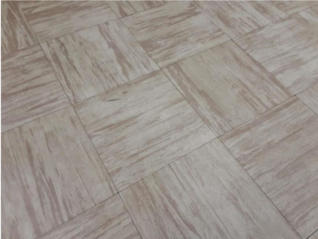
S0025A (Confirmed Asbestos), 12" beige with tan streaks, Floor, Vinyl Floor Tile and Mastic, Classroom (Location #: 59)
