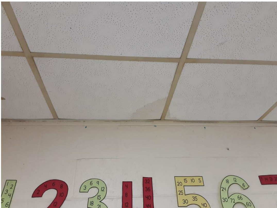
V0006 (Confirmed Asbestos), 24" x 24" pinhole, Ceiling, ACOUSTIC TILE, Ceiling Tiles (lay-in), Classroom (Location #: 71)
