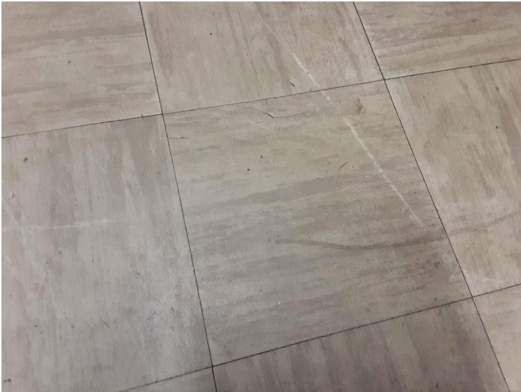
S0014A (Confirmed Asbestos), 12" tan with off white streak, Floor, Vinyl Floor Tile and Mastic, Gymnasium Office (Location #: 20)
