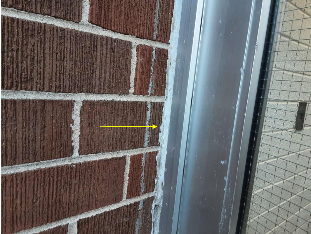
S0022A (Confirmed Asbestos), White caulking, Wall, Door, Caulking, Exterior (Location #: 66)
