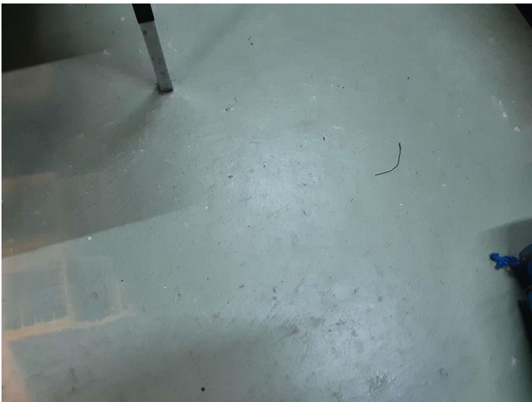
V9500 (Presumed Lead), Green, Floor, LAN Room (Location #: 7) No discreet place to sample
