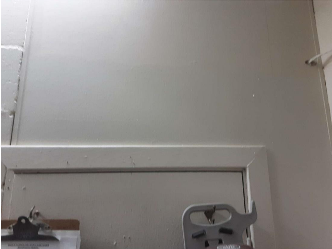
V0002 (Confirmed Asbestos), Wall, Drywall and joint compound, Custodian Room (Location #: 1)
