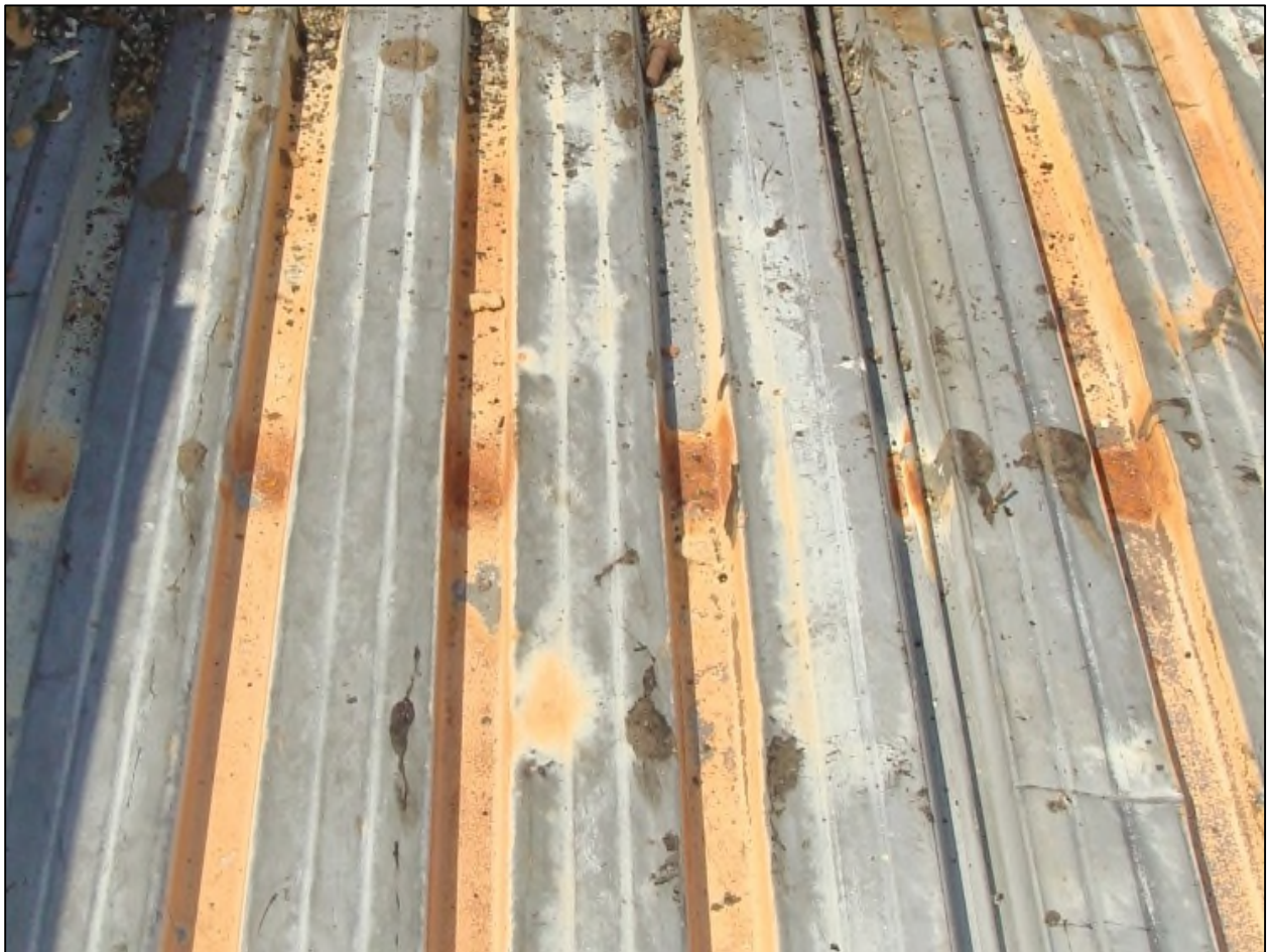
Photo of Level 2: Light to Moderate Corrosion
