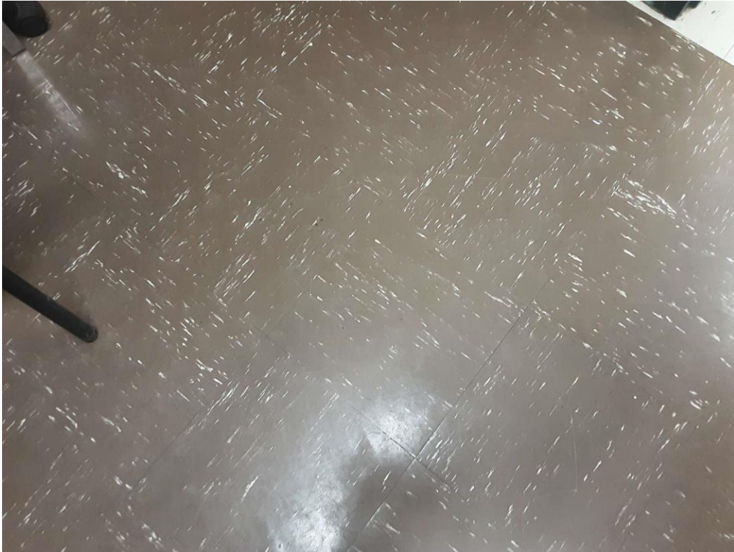
S0008B (Confirmed Asbestos), 12" brown with white streak, Floor, Vinyl Floor Tile and Mastic, Storage Room (Location #: 17)
