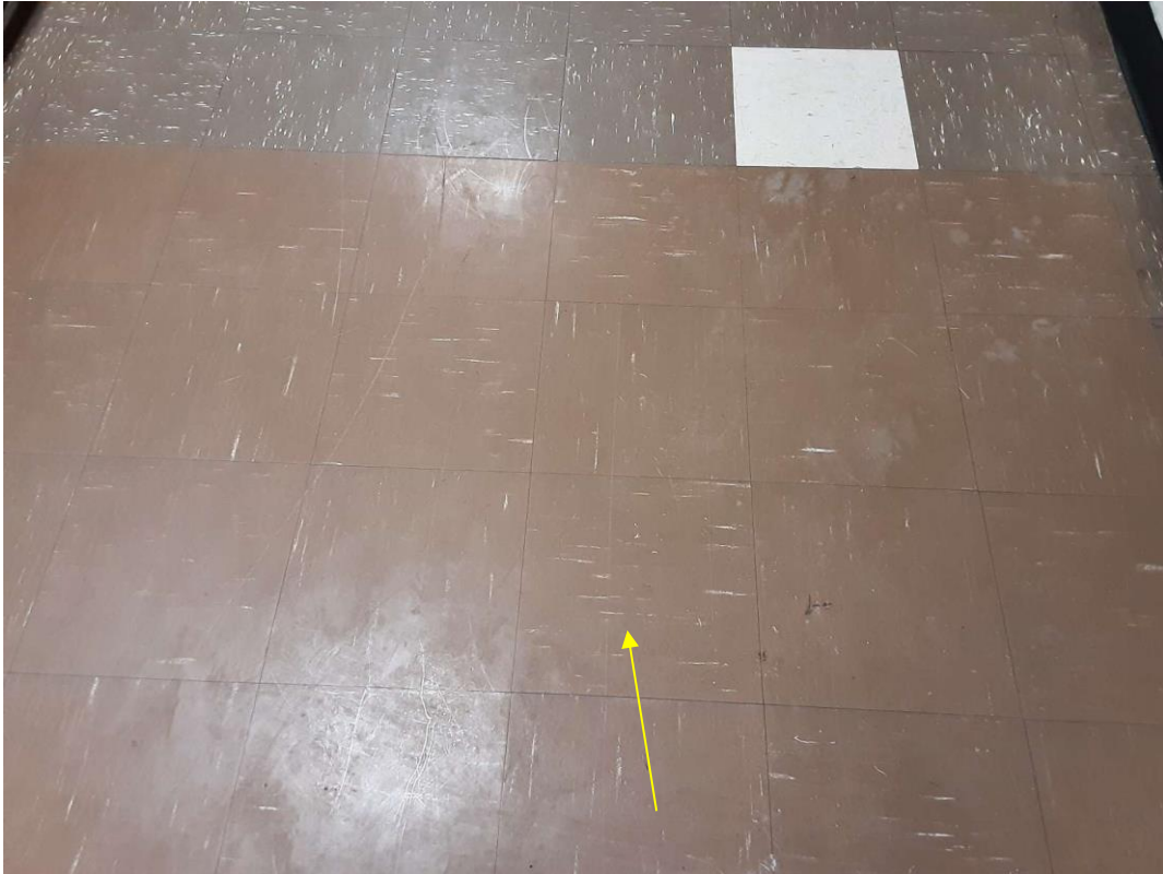
V9500 (Presumed Asbestos), 12" brown, Floor, Vinyl Floor Tile and Mastic, Hallway And Lobby (Location #: 36) No discreet place to sample
