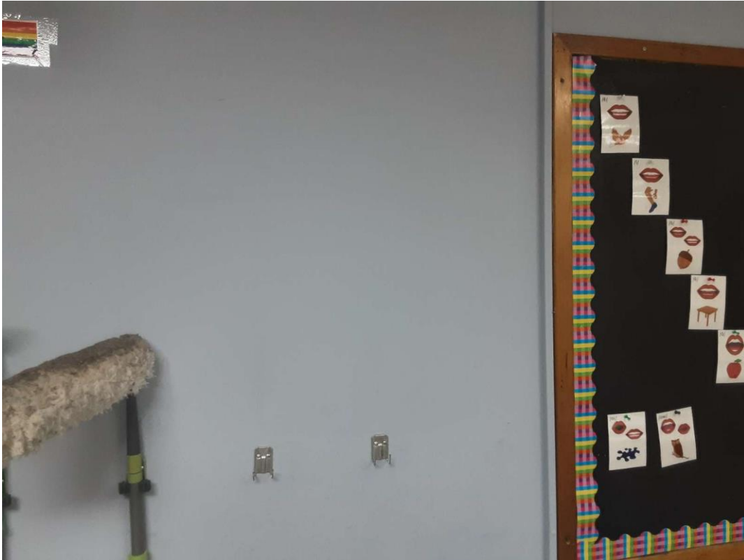
V9500 (Presumed Lead), Blue paint, Wall, Classroom (Location #: 14) No discreet place to sample
