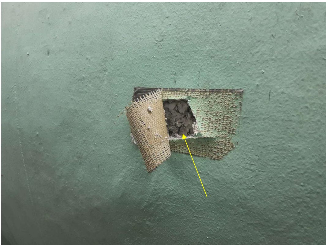
S0011C (Confirmed Asbestos), Mechanical Equipment, Heating Water Tank, Thermal Insulation, Boiler Room (Location #: 12)
