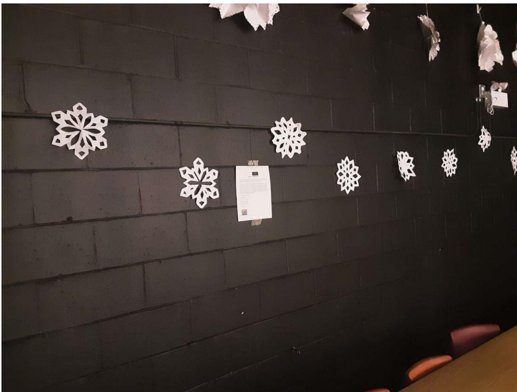
L0005 (Lead, Low), Black paint, Wall, Gymnasium Stage (Location #: 8)
