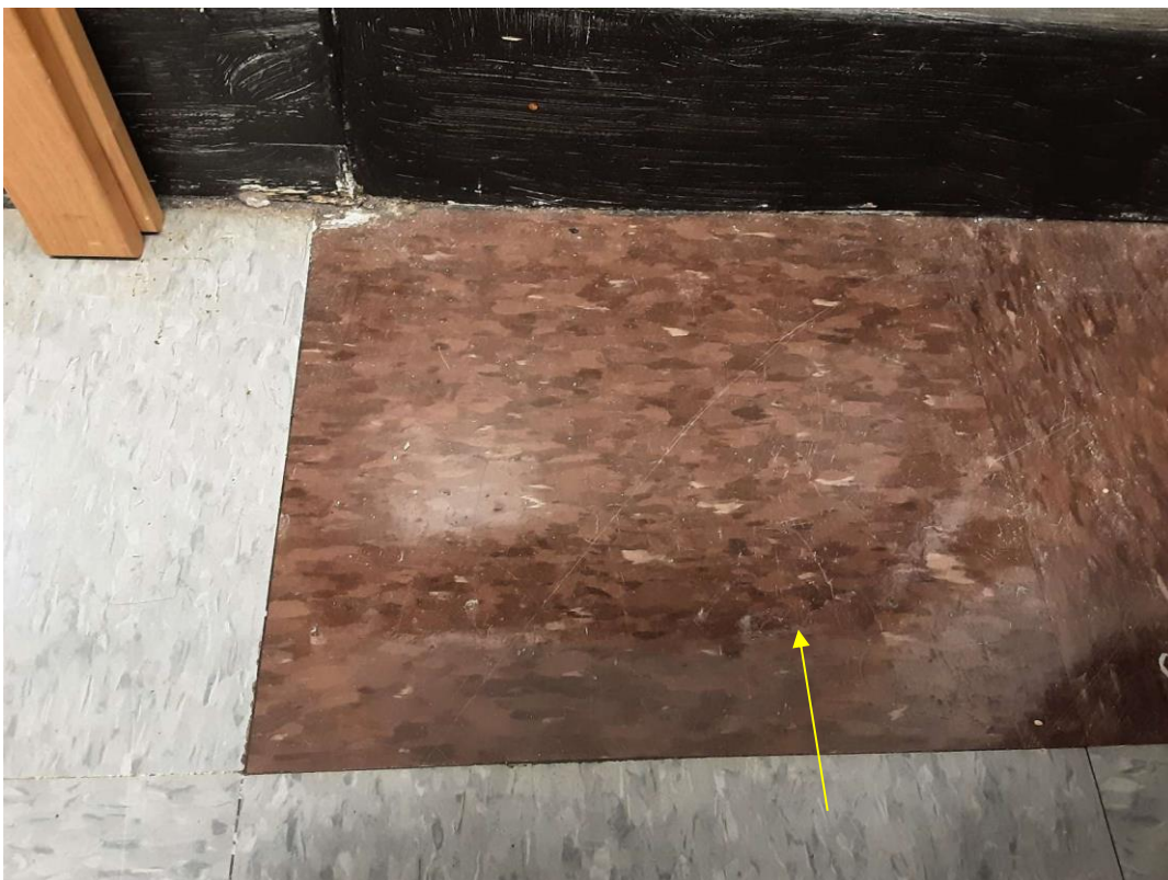
V9500 (Presumed Asbestos), 12" purple with dark purple flecks, Floor, Vinyl Floor Tile and Mastic, Staff Room (Location #: 47)
