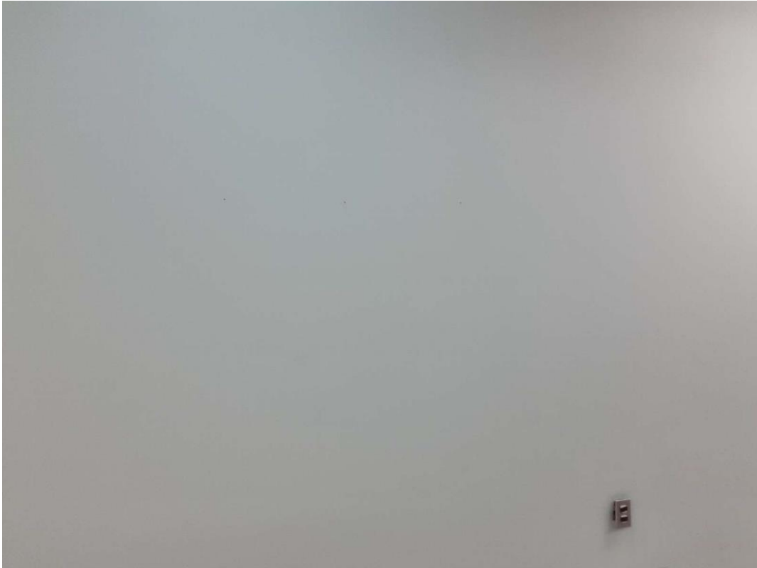
V9500 (Presumed Lead), Teal paint, Wall, Classroom (Location #: 22) No discreet place to sample
