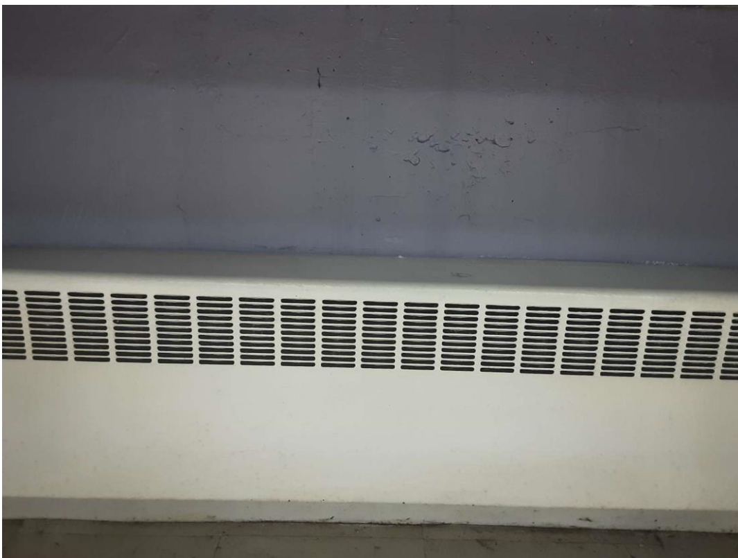
V9500 (Presumed Lead), Light purple, Wall, Classroom (Location #: 14) No discreet place to sample
