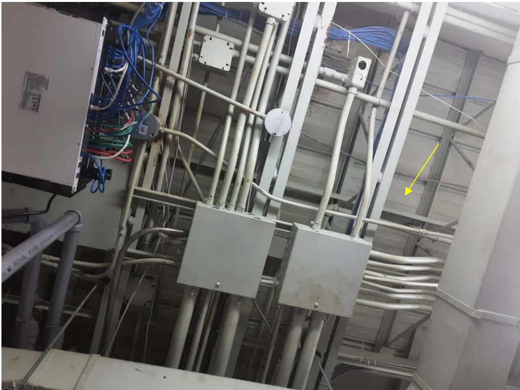
V9500 (Presumed Lead), Structure, White paint, Custodian Room (Location #: 1) Too high to sample
