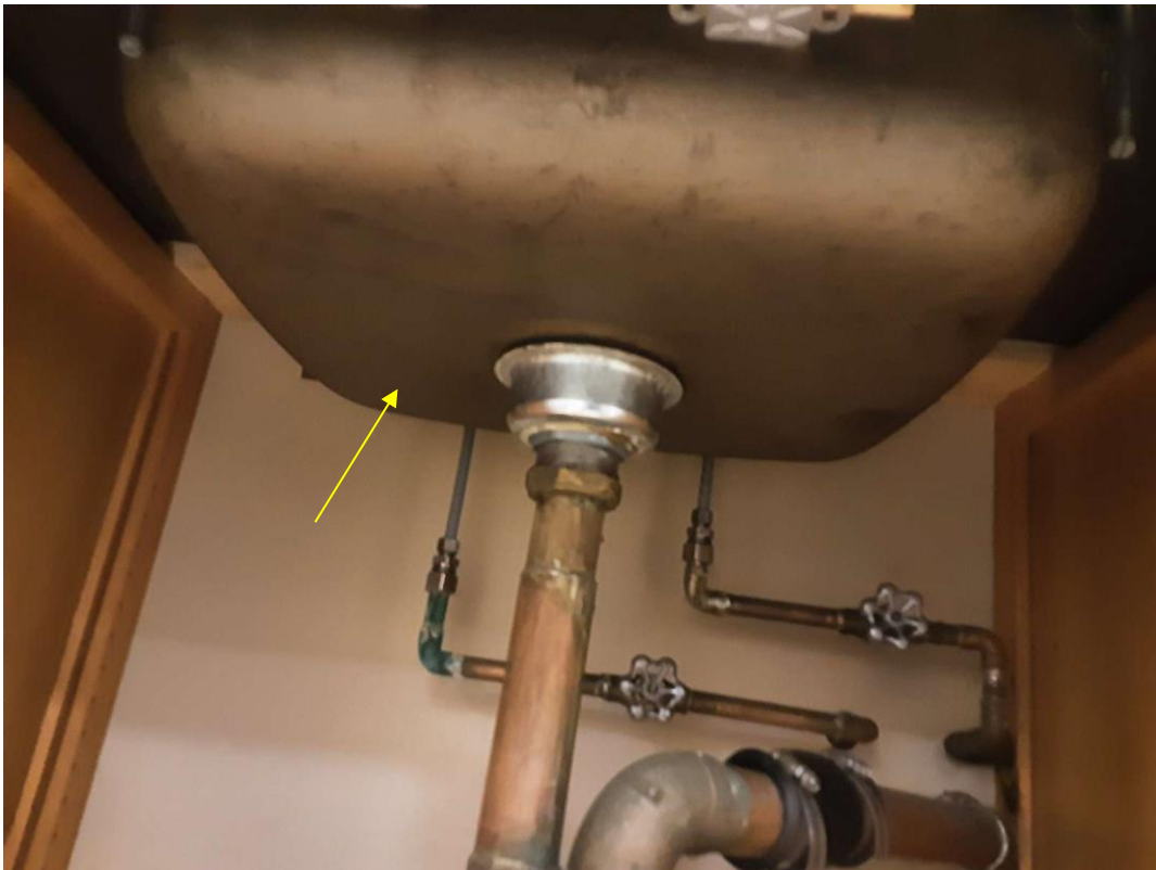
S0024 (Confirmed Asbestos), Other, Sink, Mastic, Gold, Staff Room (Location #: 47)
