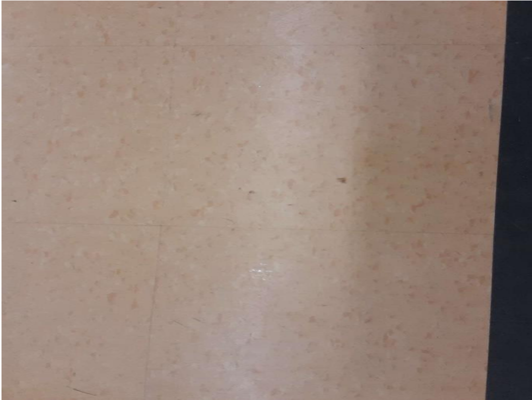
V9500 (Presumed Asbestos), 12" orange with dark orange flecks, Floor, Vinyl Floor Tile and Mastic, Gymnasium (Location #: 9) No discreet place to sample
