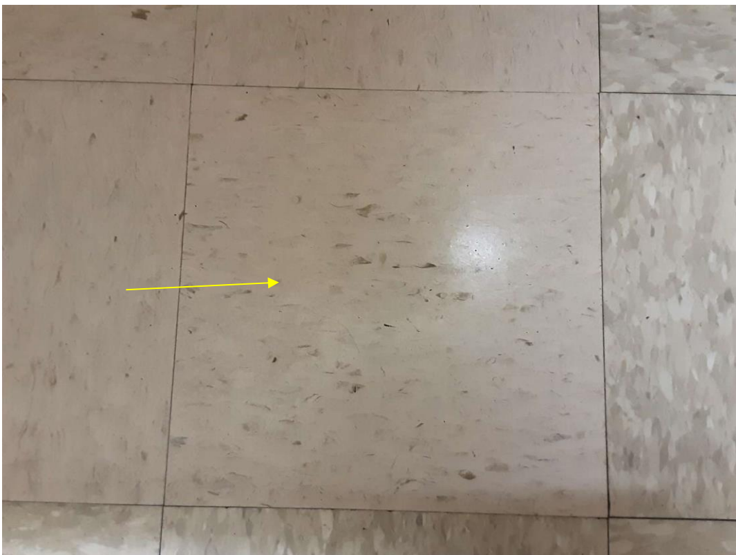
V9500 (Presumed Asbestos), 12" beige with brown marks, Floor, Vinyl Floor Tile and Mastic, Washroom (Location #: 34) No discreet place to sample
