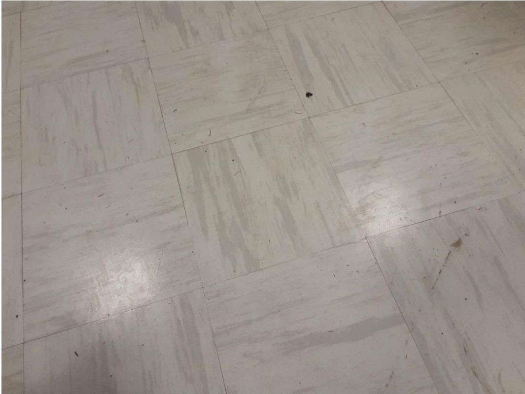
S0019A (Confirmed Asbestos), 12" off white with tan streak, Floor, Vinyl Floor Tile and Mastic, Office (Location #: 44)
