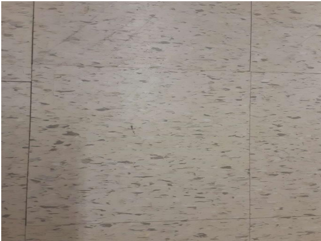
V9500 (Presumed Asbestos), 12" off white with blue and brown flecks, Floor, Vinyl Floor Tile and Mastic, Gymnasium (Location #: 9) No discreet place to sample
