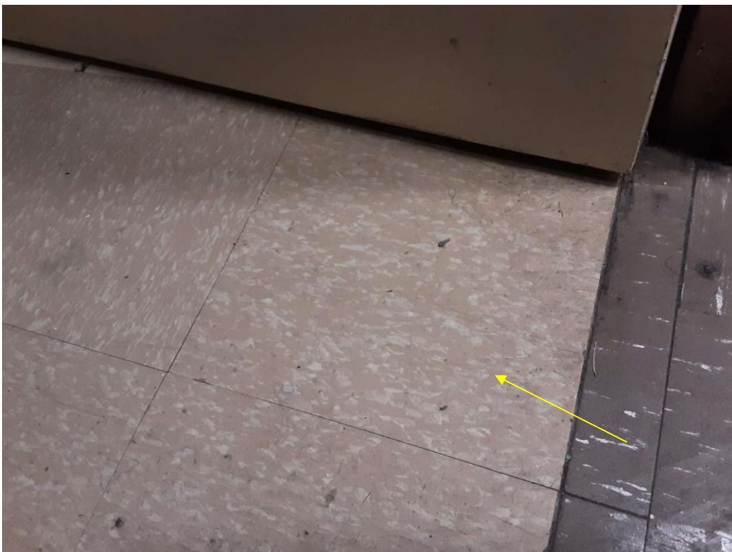
S0020A (Confirmed Asbestos), 12" peach with white flecks, Floor, Vinyl Floor Tile and Mastic, Custodian Supply Room (Location #: 50)
