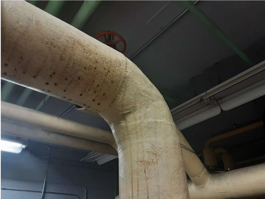
S0010A (Confirmed Asbestos), Piping, Parging Cement, Boiler Room (Location #: 12)
